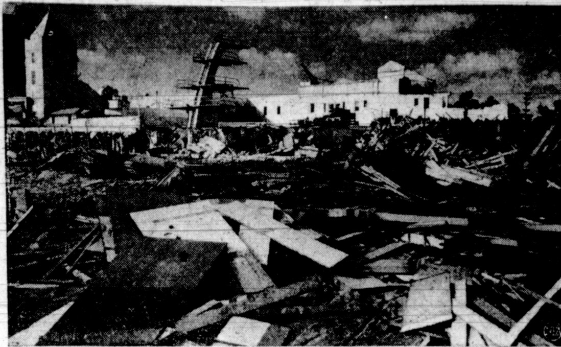
NO BOMBING, THIS—It looks like the aftermath of a blockbuster bombing raid, but this scene in Miami Beach, Fla., results from the work of professional house-wreckers. The rubble marks the fate of the once-proud McFadden-D'auville Hotel, a landmark for 30 years. Built at a cost of $508,000, the hotel spanned 500 feet of valuable ocean frontage. The late Bernard McFadden, eccentric publisher of magazines, was one of the original owners.
