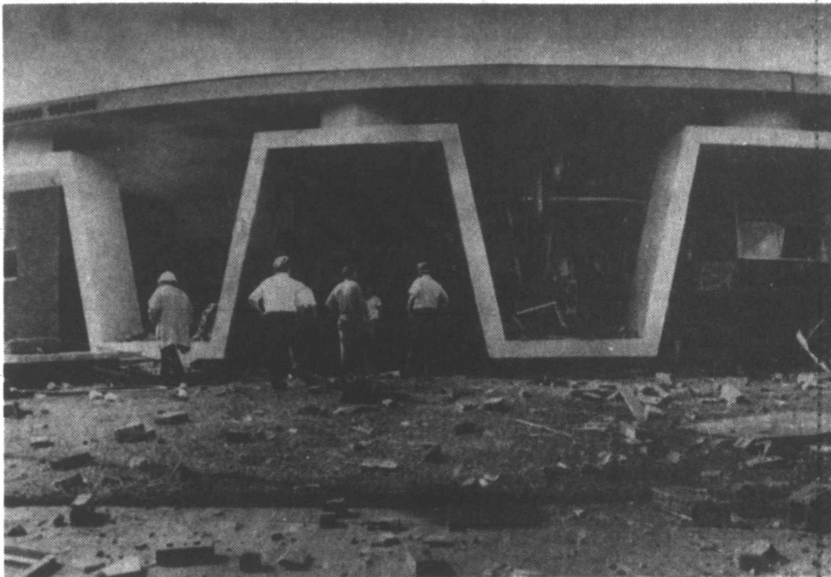
UNIVERSITY EXPLOSION — The Otho Plummer Administration Building at Lamar University in Beaumont experienced a boiler-room related explosion Thursday afternoon. One minor injury was reported. An exterior wall and one interior wall were blown away. (AP Laserphoto)
