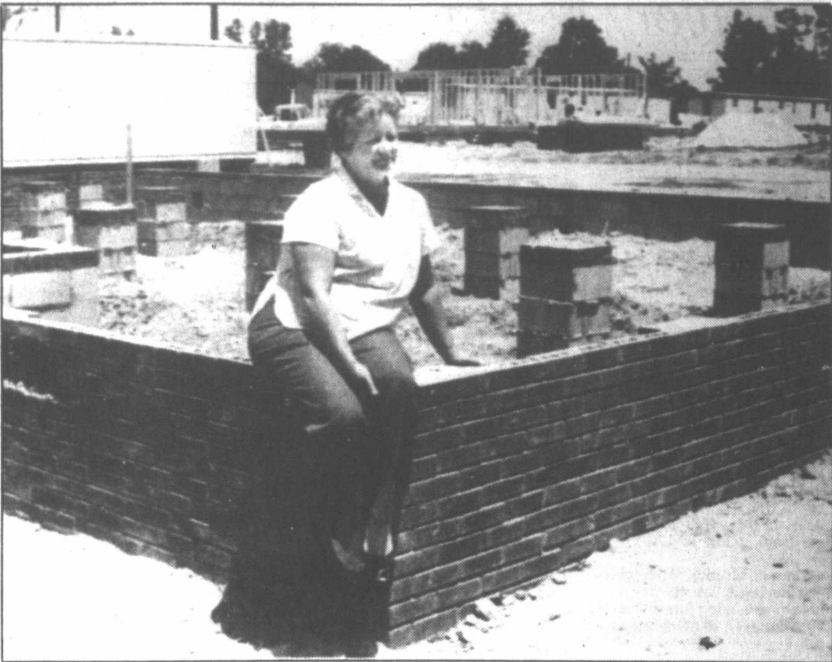
BUILDING FROM GROUND UP —Gayle Driggers of McColl, S.C. sits on the edge of the newly constructed foundation of her house in an area of the small town devastated by tornadoes
