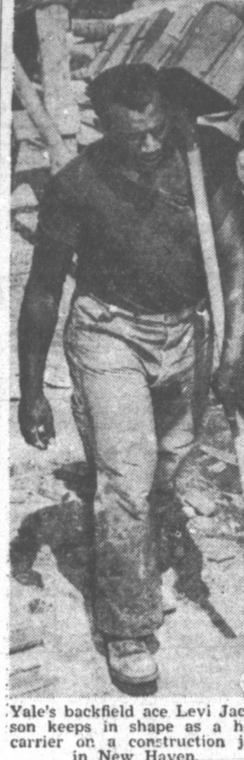
Yale's backfield ace Levi Jackson keeps in shape as a hodi carrier on a construction job in New Haven.
