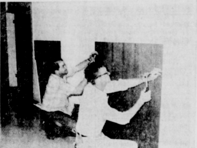
Caught with hammer and nails are Mr. C. W. Carey (left) and Mr. Miles Waldon (right) in the process of remodeling job going on at Hickman Nursing Home No. 2. Planned is much more; including carpet, new drapes, new furniture etc. Hickman Nursing Home is "The Home away from Home" and Eastland is proud of this establishment and the good service it has given, and will continue to give.
