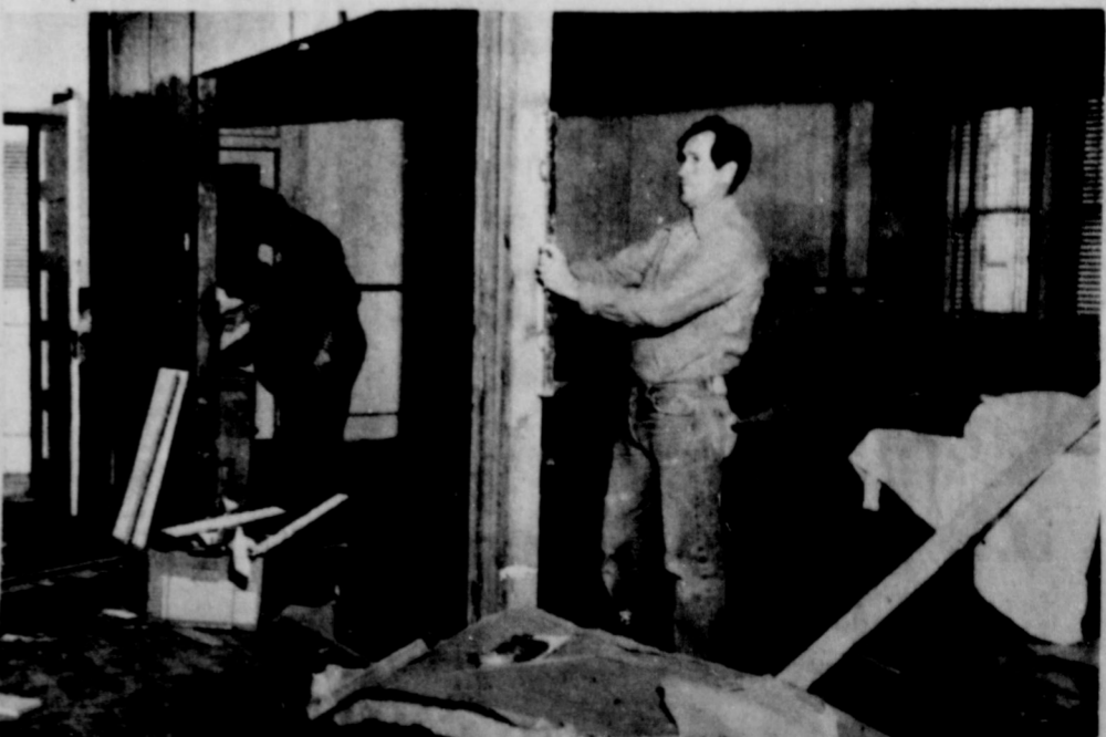
Carpenters are showing progress on the Womens Clubhouse, as the main dividing walls have been knocked out to give the Clubhouse more room and better looks.
