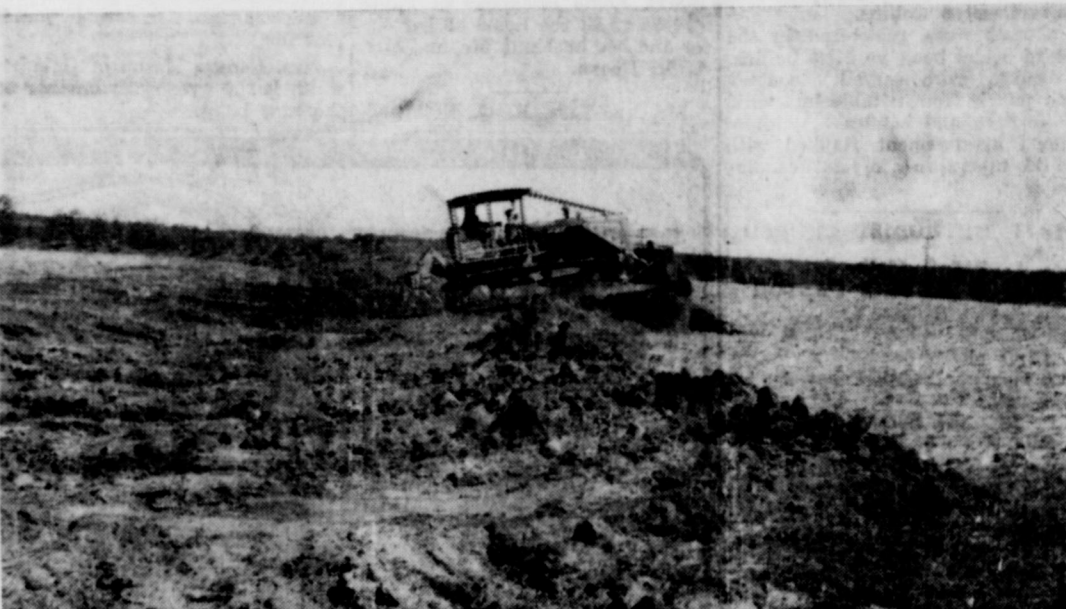
In this photo the bulldozer is making the first trip along the terrace pushing the dirt from the channel to the ridge of the terrace. Terrace channel has already been chiseled to loosen the soil.
