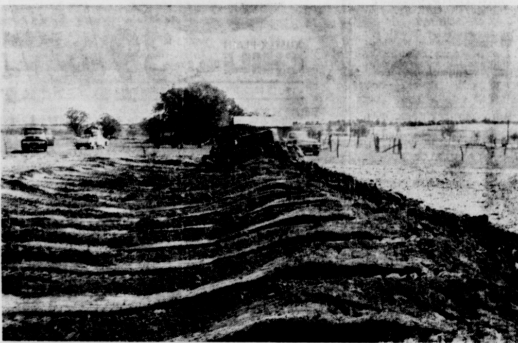
This photo shows the second trip with the dozer. The next step is the final grading of the terrace channel and bridge by running the dozer lengthwise of the terrace.
