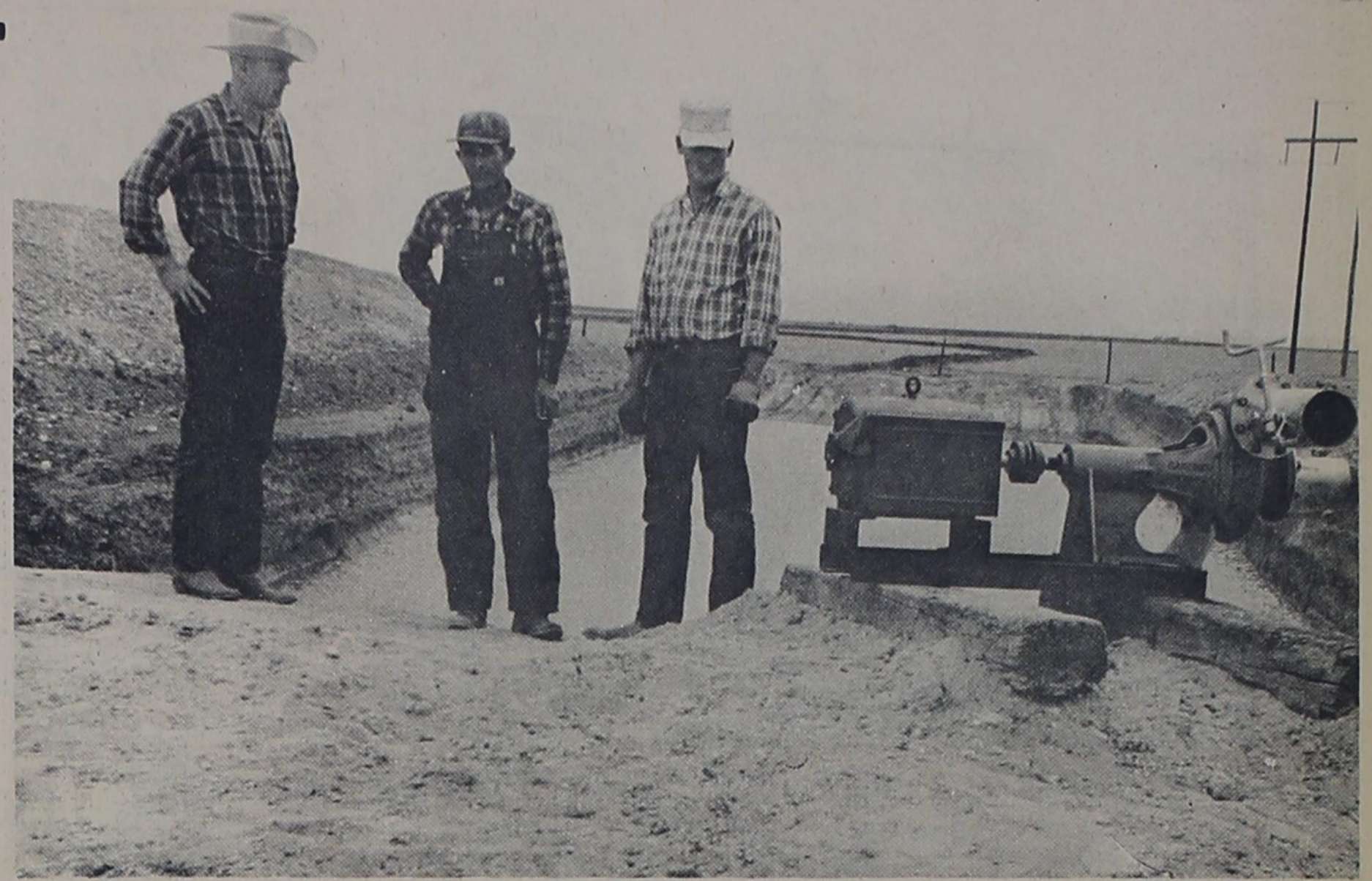
PUTTING THE FINISHING touches on a tailwater tank system near Bovina are J. D. Kirkpatrick, Buster Howard and Jim Howard. The tank is on the Jack Dunn farm, and tailwater
