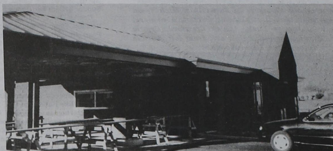
Construction of the new Muleshoe State Bank building in Farwell is coming along nicely. Its opening is expected in November.
