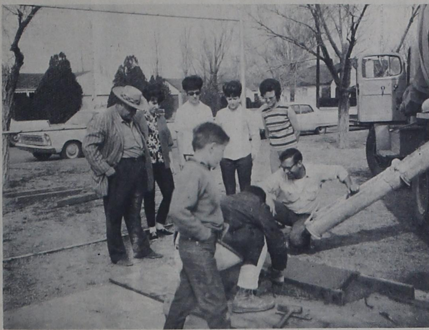
RUN TABLE FORMS -- Joe Nail, New Mexico State Highway Engineer, and Texico Woman's Club members, Mmes. Audrey Kittrell, Tommie Snodgrass, Jerri Sharp and Charlotte Pierce, look on as T. A. Autrey (Springer Corporation), and Ed Halpan, Herman Concrete Co., finisher begin work on pouring the concrete forms and uprights for picnic tables at the Texico town park.
