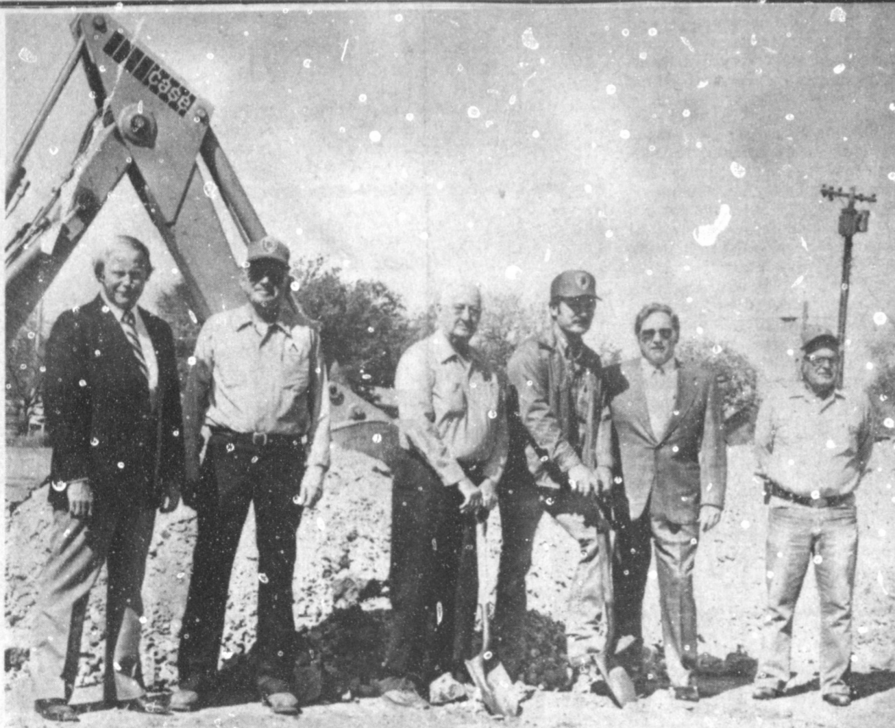
IT'S NO LONGER ONLY A DREAM AWAY--Reality set in for the Muleshoe Fire Department Wednesday afternoon when equipment was moved onto the location for their new fire station on East American Blvd. On hand for a groundbreaking ceremony Thursday morning were from left: City Manager Dave Marr; Fire Marshall Owen Jones; longtime former Fire Chief Earl Ladd; current Fire Chief Jack Dunham; Muleshoe Mayor Darrell Turner and Fire Department Captain Bob Copeland.
