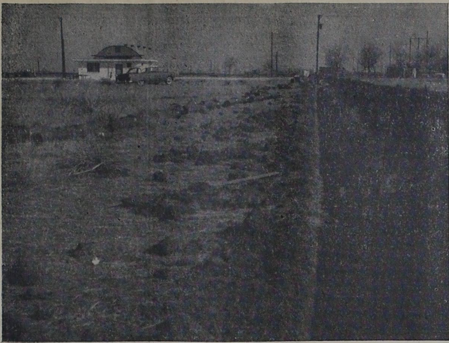
More sewer lines are being installed to serve Farwell's rapidly expanding east side. Here is a 500-foot line in the alley between 8th and 9th Streets, south of Highway 70-84.
