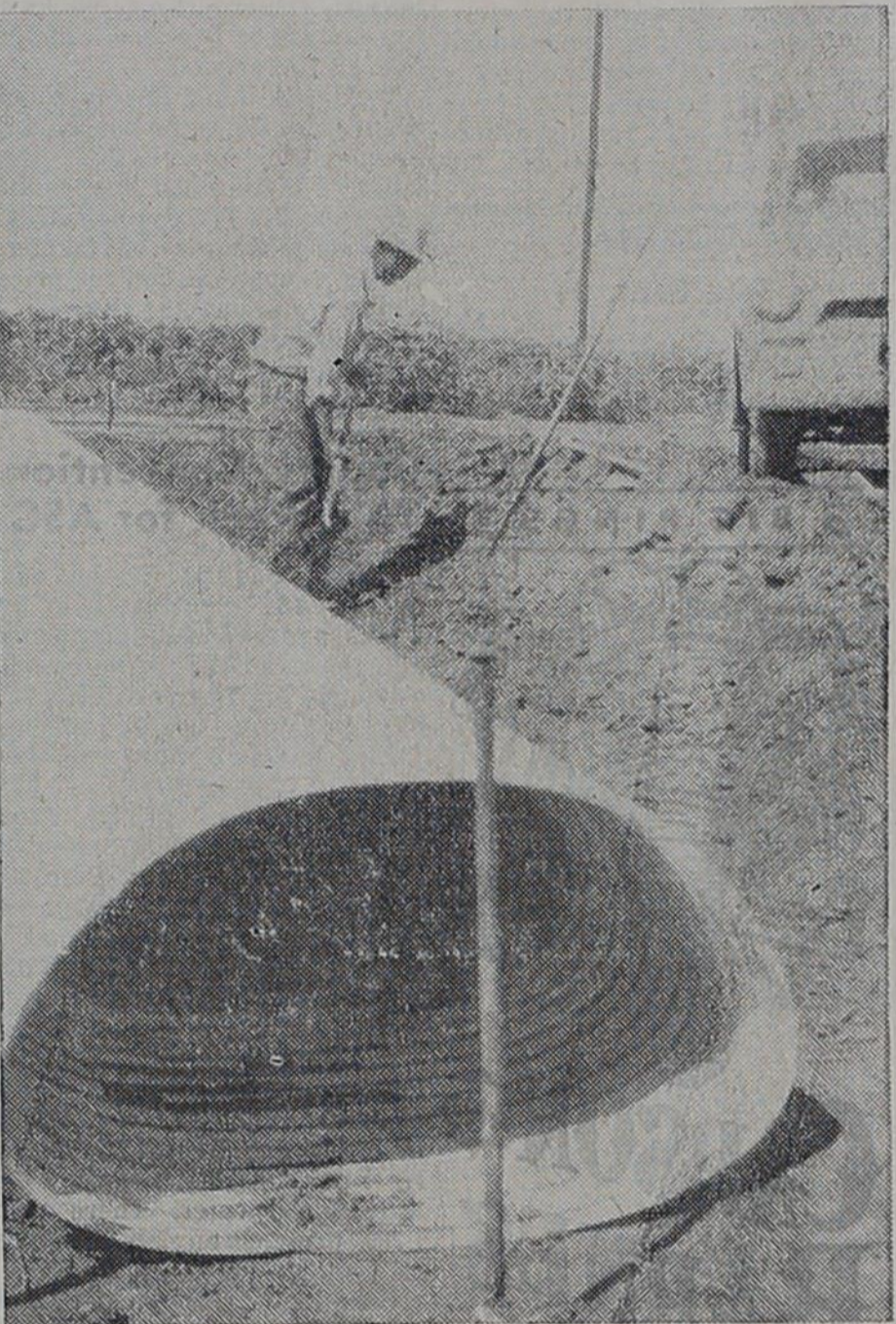
Dirt work is underway on the new Oklahoma Lane-Lariat farm-to-market road, which is due to be hard surfaced late this fall. Contractors are Kerr and Middleton of Lubbock. They also are due to complete a six-mile stretch of FM road to the Rhea community in Parmer County. The road pictured here will extend south from Oklahoma Lane, through Lariat, and join another road at the Bailey County line south of Lariat. Total length is about seven miles.
