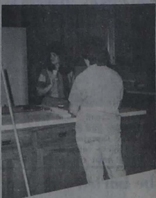
Above, Leslie Lunsford, left, and Cindy Littlejohn are taking a break while working in the new kitchen in the First Baptist Church. Below, Scott Martin, left and Gene LeClear are busy applying glue to the wall paper in the meeting room.
