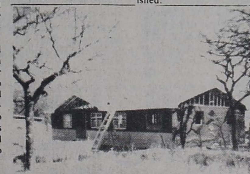
ANOTHER NEW HOME: Shown above is the new home of the Alex Granadas under construction. The new home is being built immediately behind their present home across the street from the Bruce Hirsts.
