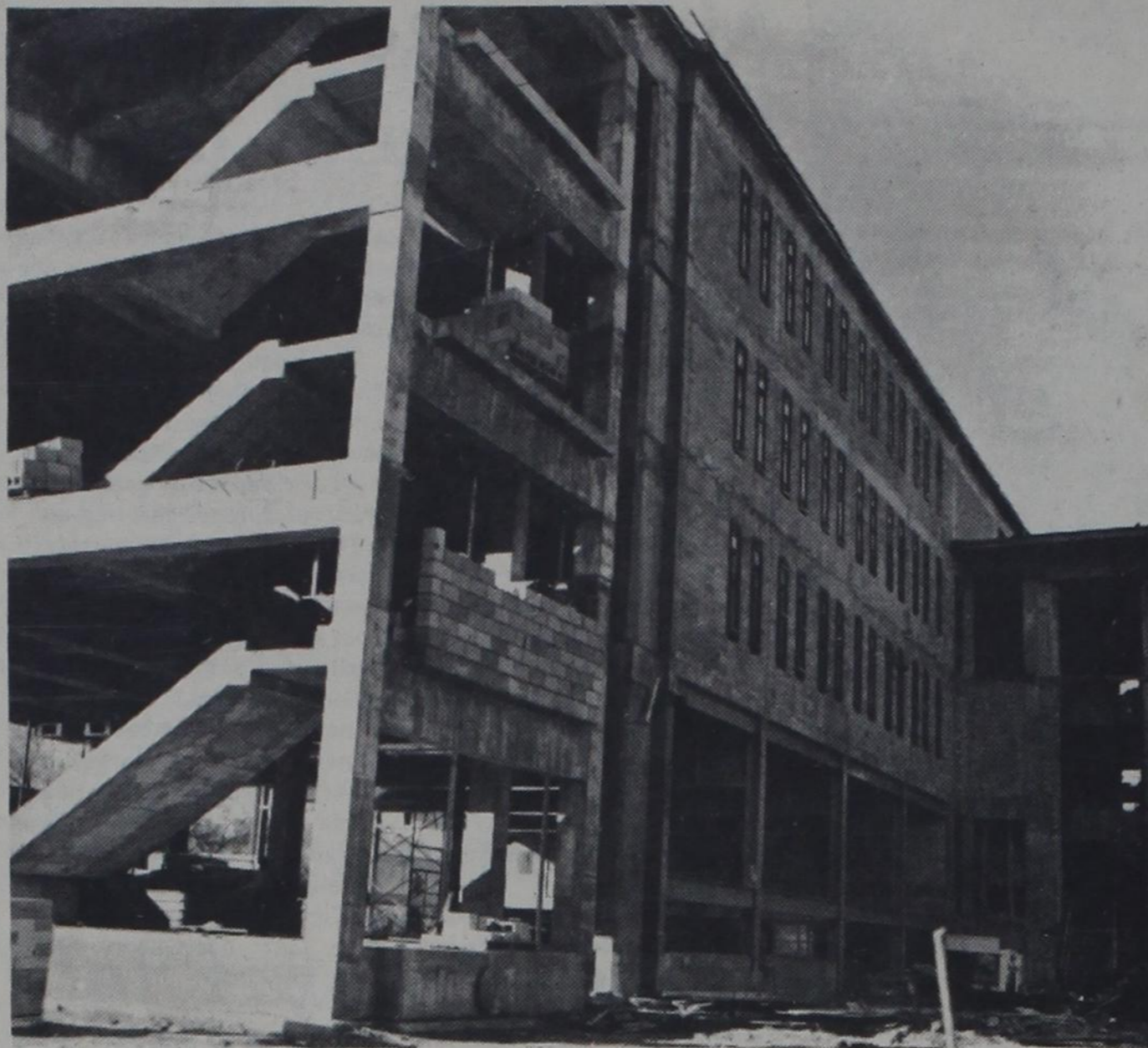
CHEMISTRY BUILDING —The new chemistry addition is 47 per cent completed. The planned completion date is Aug. 31, 1970. The building was contracted at a total cost of $5,551,078. The new structure is partially encompassed by the illustrious graffiti fence.
