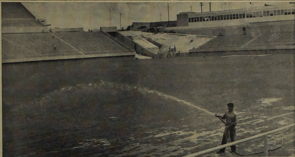
CONSTRUCTION ENTERS FINAL STAGE Preparations for the pouring of the last section of seats (upper center) began this week.
