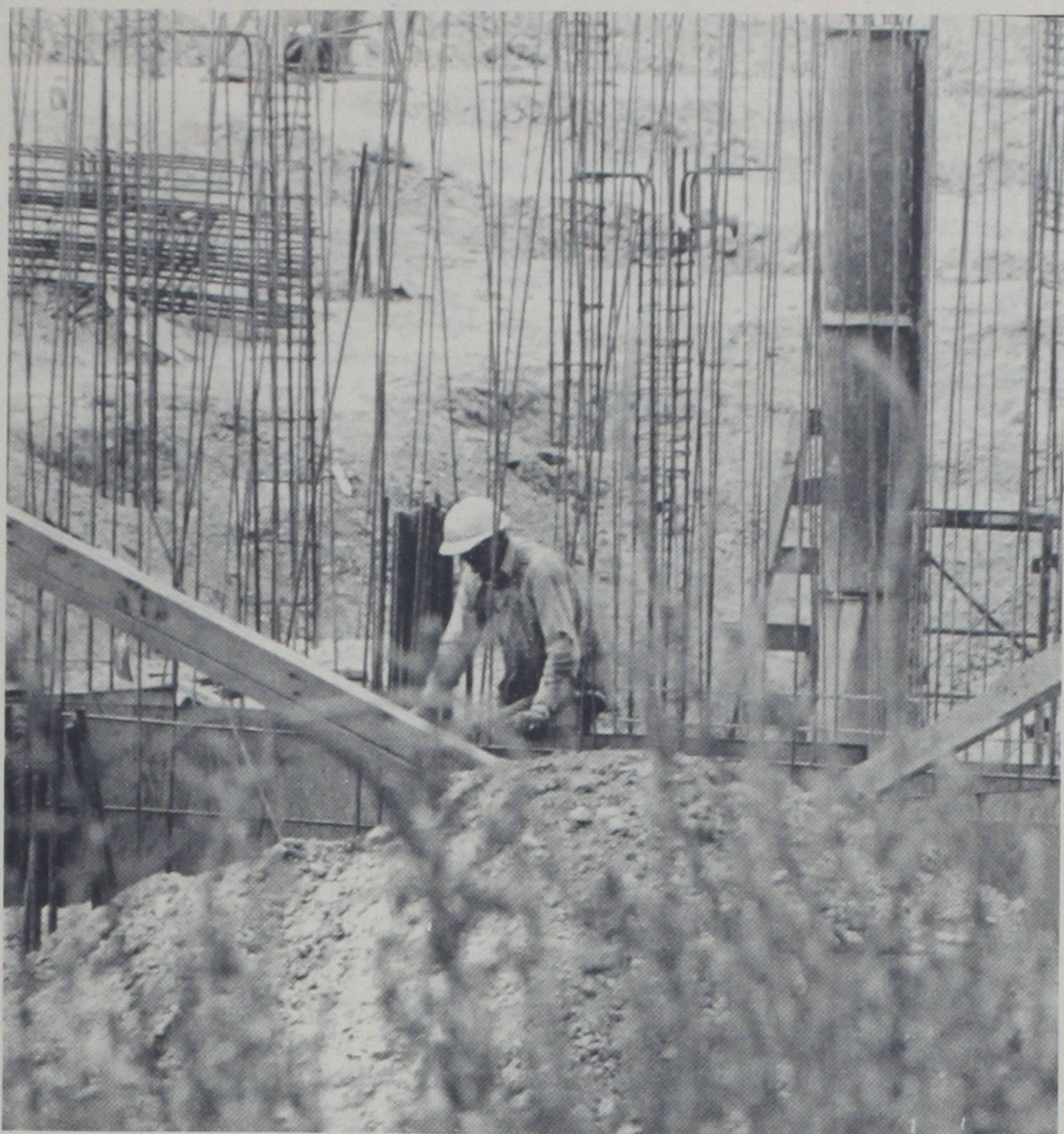
LAW SCHOOL RISES - The foundation is now being poured for Tech's $2 million Law School at its 19th Street and Indiana Avenue site. The new building, scheduled to open in September, 1969, was designed by the Dallas architectural firm of Harrell and Hamilton. The three-story structure will accommodate a projected enrollment of 600 students and can be increased to serve more than 1,000. (Staff photo by Milton Adams)
