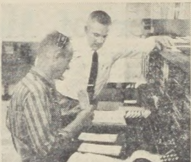
"9:10 a.m. The State Police at Andover have reported trouble with a mobile radio telephone. I discuss it with the test deskman. Naturally, we send a pairman out pronto to take care of it."
