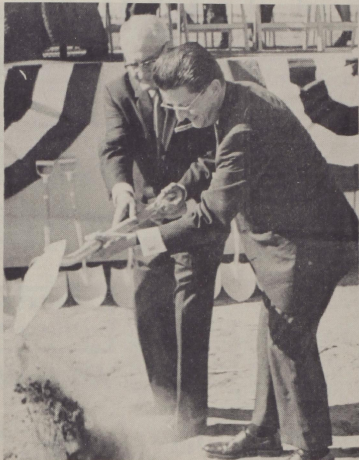
GROUND BREAKING — Turning the first shovel of dirt for the new Lubbock State School are Jess M. Osborn, of Muleshoe and the Texas Board of Mental Health and Mental Retardation
