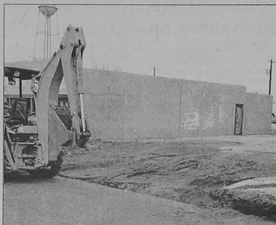
GROUND BREAKING for the new EMS facility is completed. Located next to the clinic, the land was donated by the City of Matador. Completion is projected for May, 2008.
