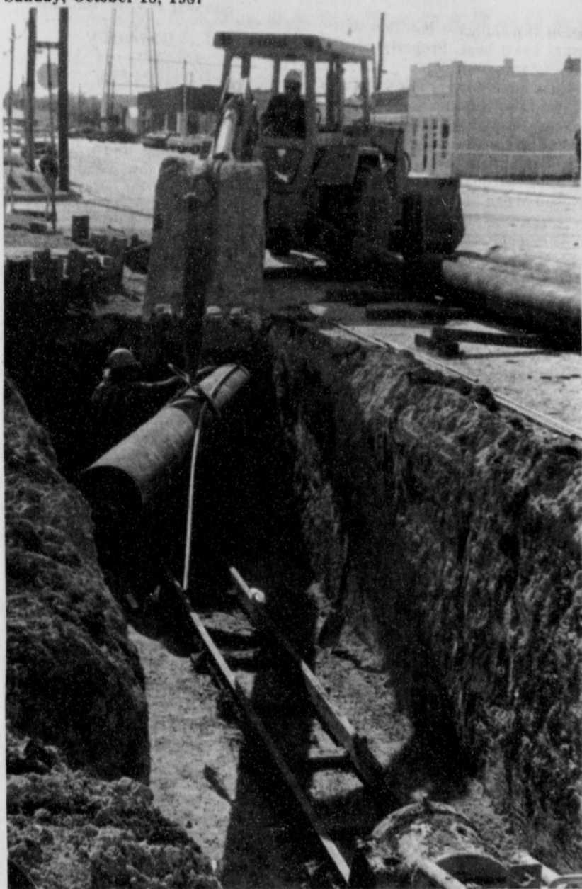
WHAT, NO POLES? . . . Spearman telephone users will shortly be utilizing a new fiber optics telecommunications system being installed underground here by GTE.
