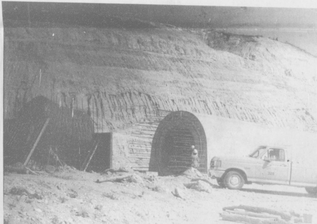
The 11 foot diameter pipe that will serve as the normal lake level spillway, nears completion. The concrete tunnel will have walls 40 inches thick. This spillway, on the West end of the dam, is known as "Morning Glory."
