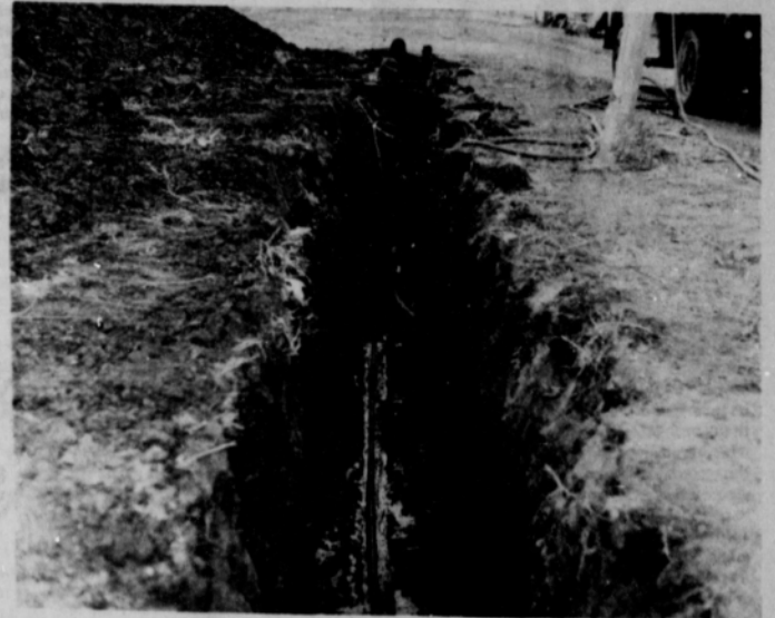
Here's how the opening under East Seventh Street was made by this crew of three from Amarillo, Edward Florez, Alfredo Mata and Juan Flores, in a form of tug-of-war put their weight behind a rotating bit, pulling it through the ground to create the hole for the eight-inch pipe.
