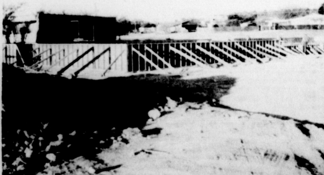
CONSTRUCTION OF NEW NURSING WING progresses right on schedule. Foundation work is under construction here. Forms are in place and almost ready for concrete. Construction is at the north end of the Crockett County Hospital which may be seen in background at left. Homes in the Henderson addition of Ozona may be seen in the far background.
