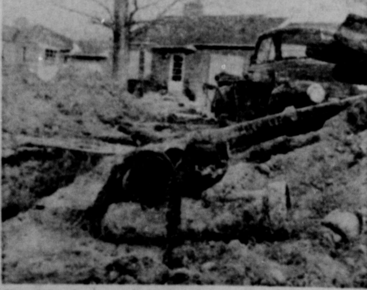
Illustration from new homeowner booklet on house sewer failures shows lawn havoc caused by removal of 70 feet of non-metallic pipe infested with tree roots—note root-clogged pipe in foreground.
