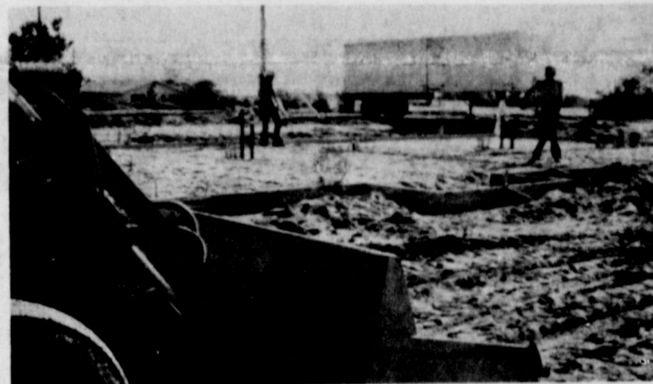
Work is going full swing on the McLean Housing Authority apartments being built on the northwest side of town, with foundations poured this week. The complex will include eight apartment units. Construction is expected to be finished in five months or less. (Staff Photo)
