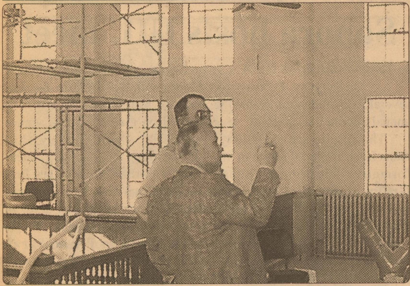
There used to be a balcony right up there — County Judge Johnny Griffin and Commissioner Johnny Mayo discuss renovations to the courtroom on the 2nd floor of the Schleicher County Courthouse. Griffin noted that demolition had revealed where an old balcony had once been in the back of the courtroom
