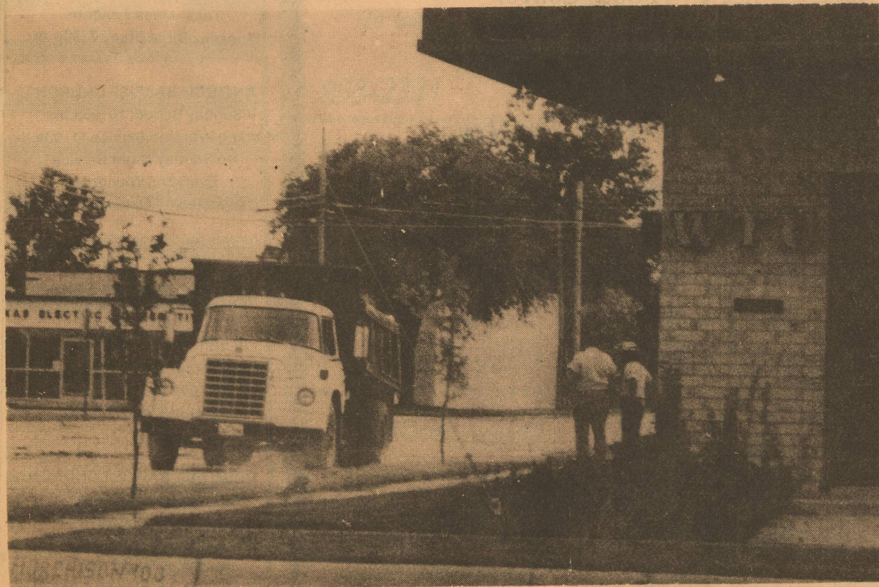
City had begun paving work in front of the Post Office. The process should be complete within a week barring rain.
