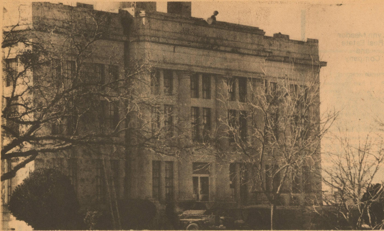
The Schleicher County courthouse gets a re-roofing job this week. The workmen have a good view of Eldorado from their high perch.
