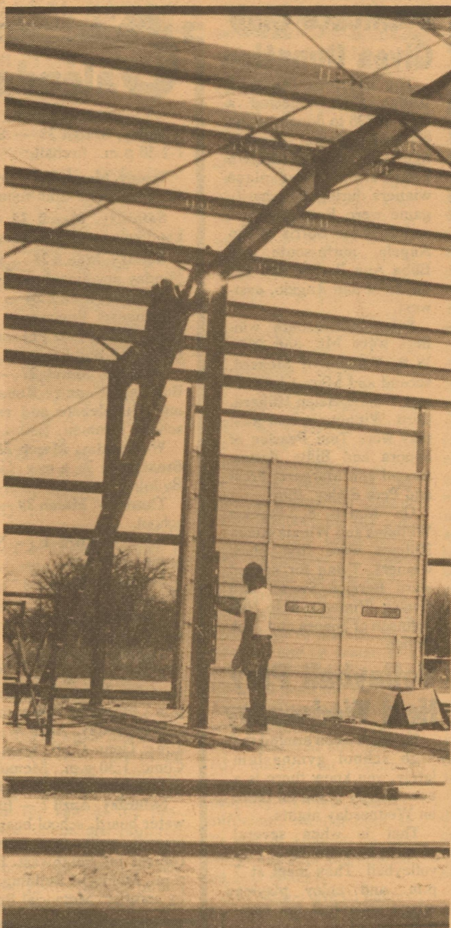
SPARKS A' FLYIN' — A workman is busy welding a brace on the construction sight of the H. G. Automotive next to Western Auto, while a co-worker watches. The business is scheduled to open in mid-April, depending on weather.
