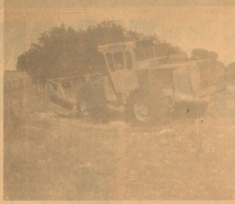
on display recently on the Mort Mertz ranch south of Eldorado to show its effectiveness in clearing land. At left, is brush before the machine began
