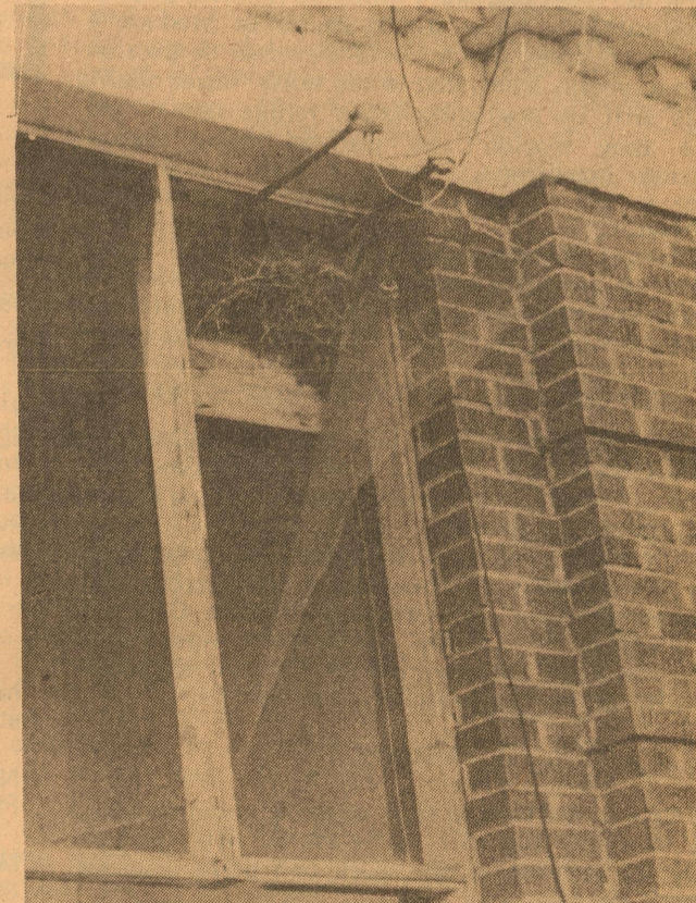
Bird nests, such as this one, could create a fire hazard.
