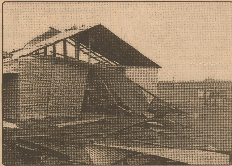
photo by Kathy Mankin Twisted sheet metal — This barn, belonging to W.F. Edmiston was severely damaged by an apparent tornado, spawned by a line of storms which crossed the county Wednesday, April 19th.
