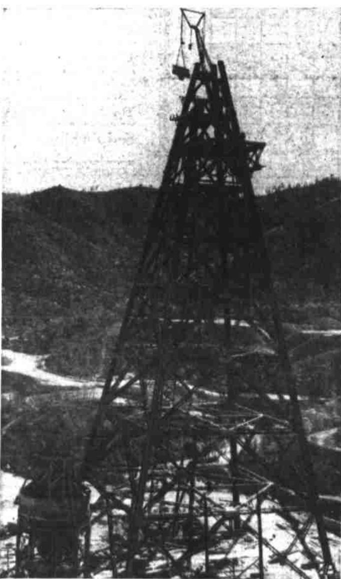
DESERT SKYSCRAPER —From this 460-foot tower will suspend the seven cables anchored at key points surrounding Shasta dam, California, thus providing seven inclines over which concrete-bearing buckets will glide. Shasta dam is being built by the U. S. Bureau of Reclamation to control the water and power of the Sacramento and San Juan rivers.
