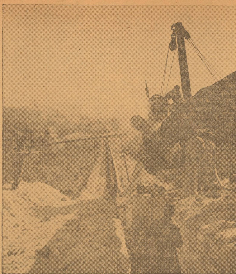
PROTECTIVE COATING of enamel, glass fiber and asbestos felt wrappers are applied to the 24-inch diameter Rancho Pipe Line in a continuous operation by an ingenious machine, right, just before being lowered into the ditch. A pad of soft earth, free from hard objects, is used to cushion the pipe in rocky areas. A pipe so protected lasts for years without corroding or wearing.
