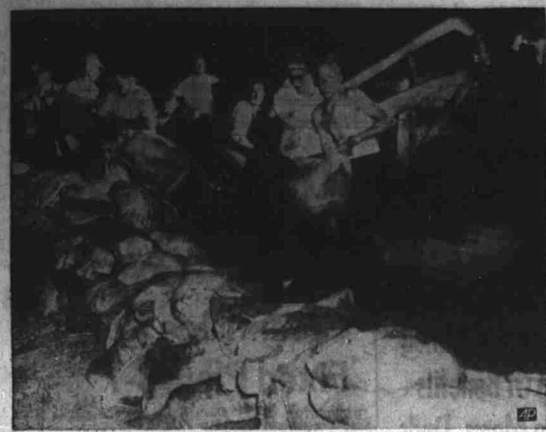
Men and bulldozers worked through the night in Des Moines, Iowa, to build a sandbag levee along the east bank of the Des Moines River in the heart of Iowa's capital city. Some 200 volunteers, including some women and children, filled, tied, loaded and piled the bags as the river rose past the high set in 1947's disastrous flood in Des Moines. The Weather Bureau said the river crest was just over 30 feet. (AP Wirephoto). (See Story Page 1).
