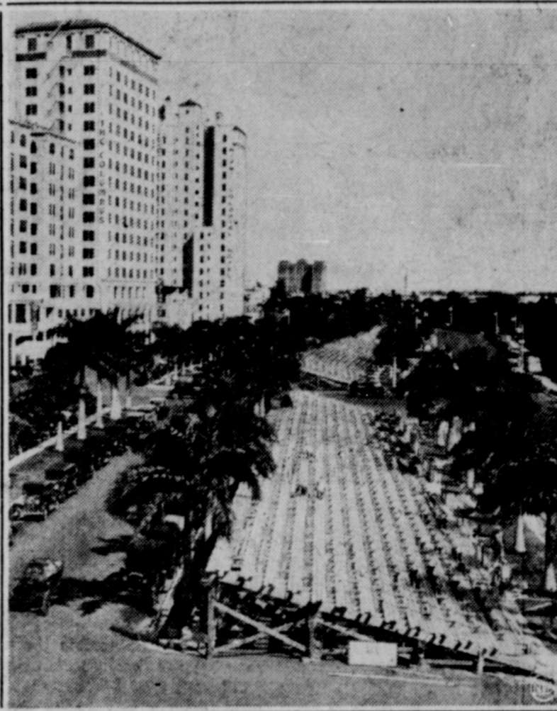
The climax of the American Legion's national convention in Miami, Fla., will be reached October 23 when the annual big parade will be held. The huge grandstands, shown above in course of construction along Biscayne Boulevard, will seat thousands of spectators. More than 100,000 World War veterans are expected to attend.
