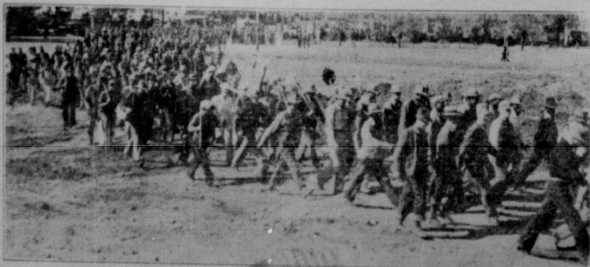
Three thousand men are working each day on the huge lot of the Texas Centennial Exposition in Dallas. Three shifts a day speed work for the opening date, June 6. Above workmen are shown filing in for the late afternoon trick. As the Exposition, federal, state, city and exhibitors' building schedules develop, more men are hired daily, further cutting into the fast vanishing ranks of Texas' unemployed.
