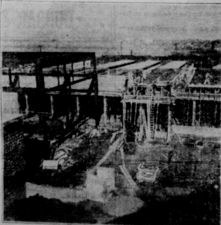
This photograph gives a realistic idea of how rapidly work is progressing on the Texas Centennial Exposition's huge lot in Dallas. All of the frameworks shown above are part of Livestock Building No. 2, one of two structures which will house the greatest stock show the United States has seen. The two buildings, their construction cost close to $400,000, will contain an ultra-modern veterinarian hospital.
