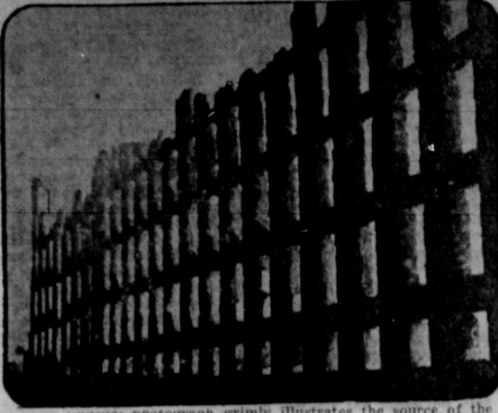
This unusual photograph grimly illustrates the source of the $25,000,000 fire which wiped out part of the business section of Fall River, Mass. The blaze started behind this wall of the Poesset Mills. Fire companies from many neighboring cities were hampered in their work by a freezing gale.
