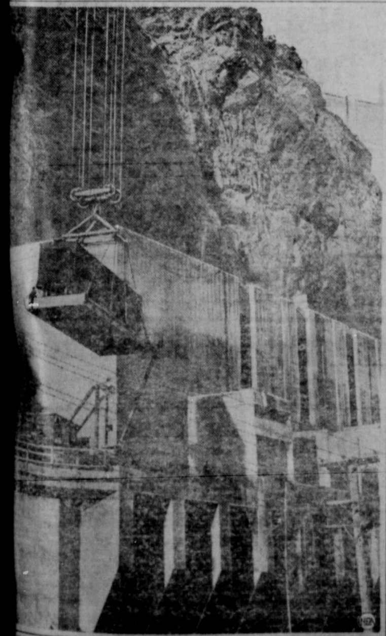
They're still doing big things in their accustomed big way at Boulder Dam—lowering a loaded steel box car 800 feet into Black Canyon to the runway of the Nevada powerhouse in this unusual picture. Note that a workman has accompanied the car's dizzy descent. The 150-ton cableway is a part of the permanent transportation system to the powerhouses at the foot of the dam, the crest of which may be glimpsed upper right.
