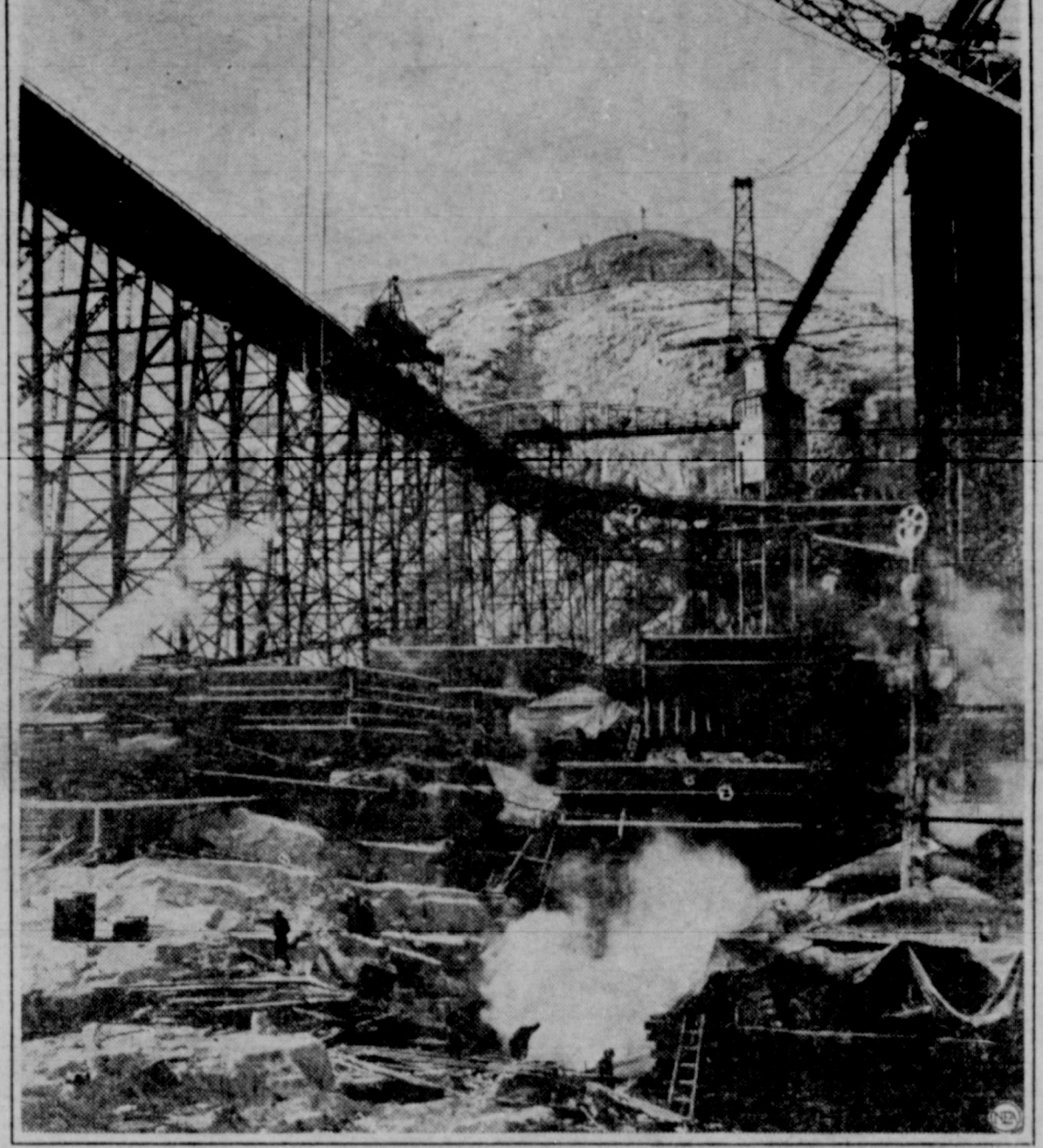
While the shivering and snow-capped heights above the Columbia's river bed look down on them, workmen pour concrete into steam-heated workings of the rising Grand Coulee dam. The canvas cover at lower right with steam leaking out from it protects a new pouring from freezing before it sets. Irrigation, navigation, power production are all to be promoted by completion of the dam, the builders of which have felt a spur in the U. S. Supreme Court's interpretation of the TVA case.
