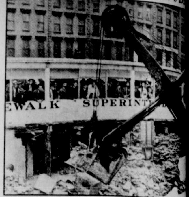
Here's first national convention of Sidewalk Superintendents. People who gather to gape for hours at a steamshovel. For the meeting was special platform from which delegates over excavation work at Rockefeller Center, New York.
