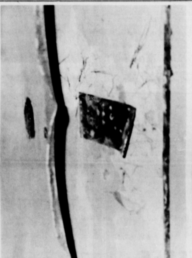
THE DOOR TO THE SAFE in the Springlake High School office was badly damaged in Sunday night's break in. However, thieves were unsuccessful in their attempt to open the safe door.
