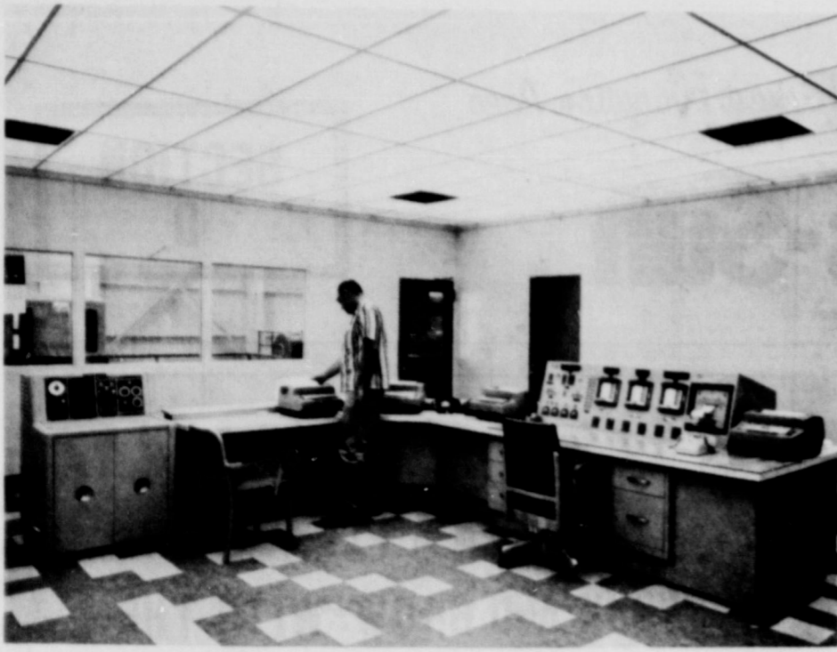
THE CENTRAL INFORMATION CENTER in the control room at Plant X, Southwestern Public Service Company's largest generating station, provides the control room operator with 400 different items of information about the plant every two minutes. The equipment includes from left to right, the automatic dispatching console, data loggers, a sequence recorder and a digital computer. The information provided by the recording and logging equipment makes it possible to operate the plant in the most efficient and economical manner at all times.
