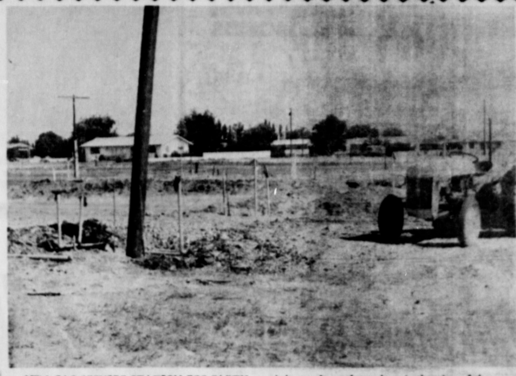
NEW GAS SERVICE STATION FOR EARTH... A busy place these days is the site of the future home of the El Paso station, east of the La Casa Motel. Plumbing is being installed by Brady Plumbing Co. of Lubbock.
