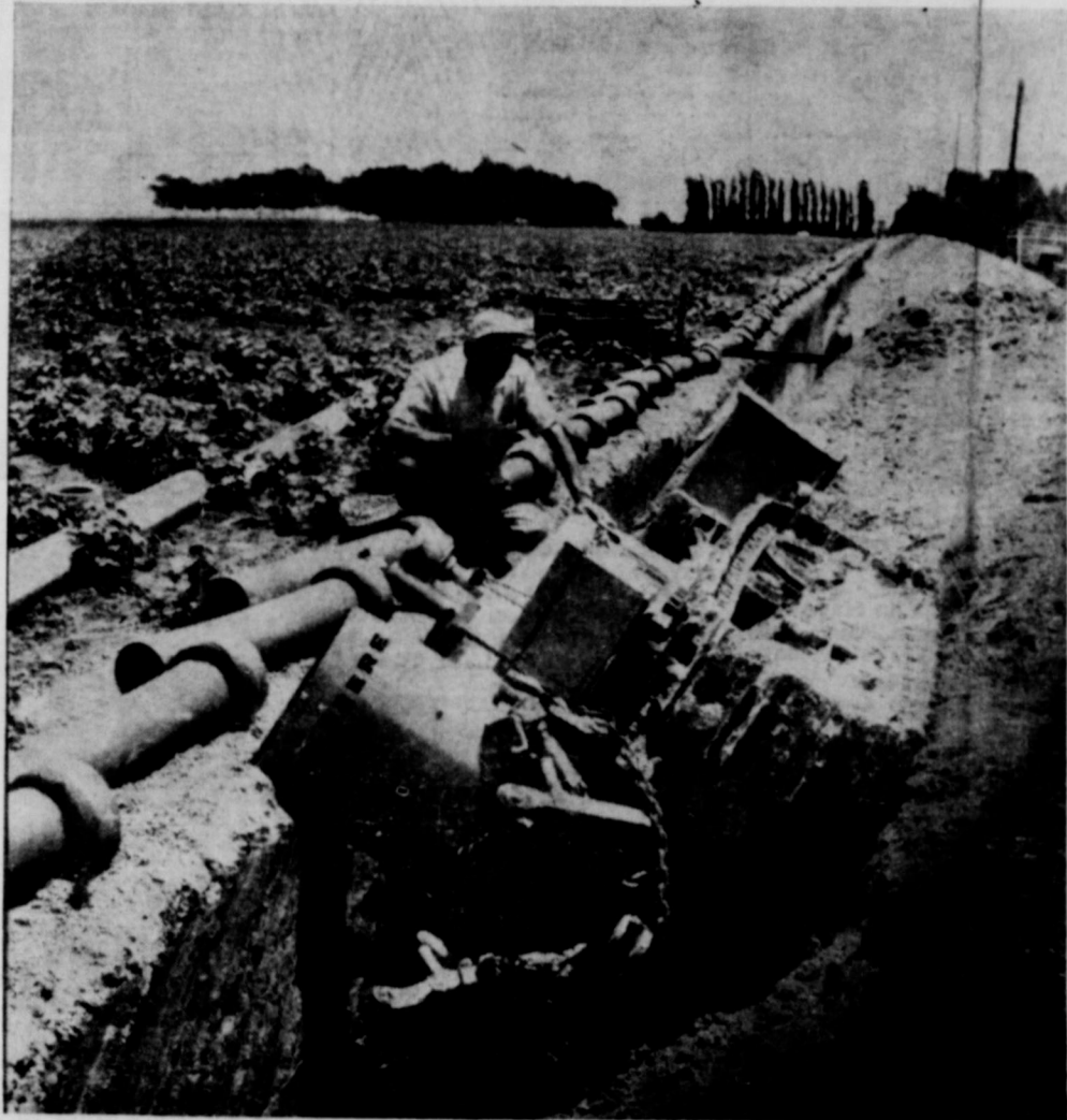
DEEP IN THE HEART OF TEXAS (SOIL). — This Bulldozer driven by Luther Vaughn Contractor for Earth's Water-Sewer Improvements fell into the 8 ft. sewer ditch as the surface gave way, caving in as he was covering up the ditch. Vaughn escaped injuries as he was thrown free of the falling bulldozer.
