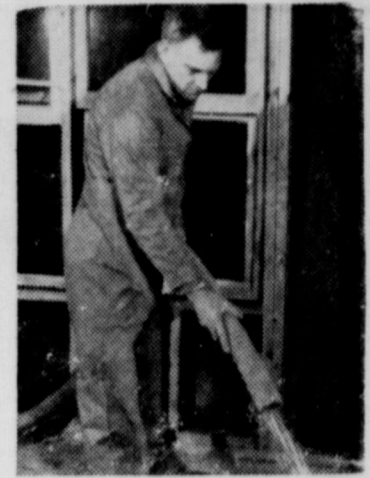
Workman installs mineral wool insulation in attic floor of an older home, using "blow in" system. This method, developed especially by mineral wool engineers to make insulating existing houses easier, employs air pressure to force the insulation into hard-to-reach wall spaces, floors, and ceilings.
