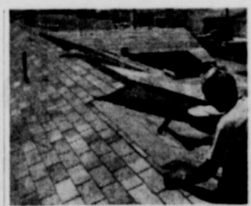
Roofer applies asphalt ridge shingles on roof of new home to provide maximum protection and good appearance.
