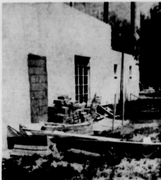
THIS CAN BE PREVENTED --- Old lumber and bricks are shown on the south side of the fire station, marring the alley approach. Will this situation be remedied? This block, and adjoining blocks on Main Street, have a number of such sights, which, when removed, will greatly improve the appearance of city streets and alleys.
